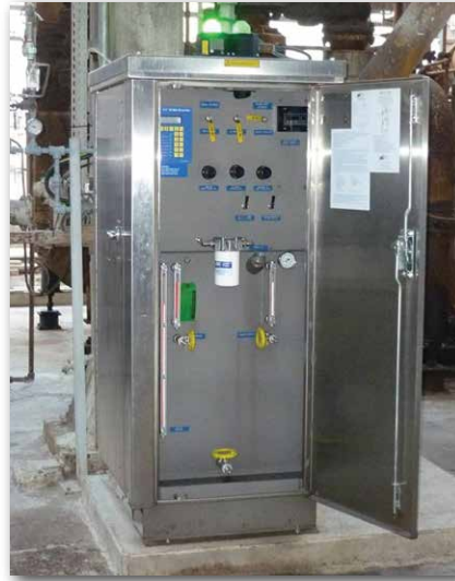
Figure 7: IVT oil mist lubrication console in No. 3 Topping Unit at Raffineria di Milazzo
