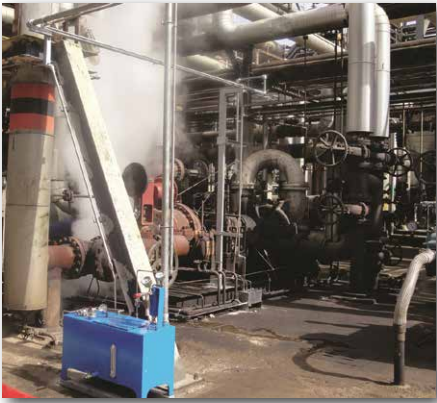
Figure 3: Oil mist lubrication demonstration with a small portable oil mist generator. The centrifugal pump is driven by a steam turbine. Free steam explains oil contamination risks.
