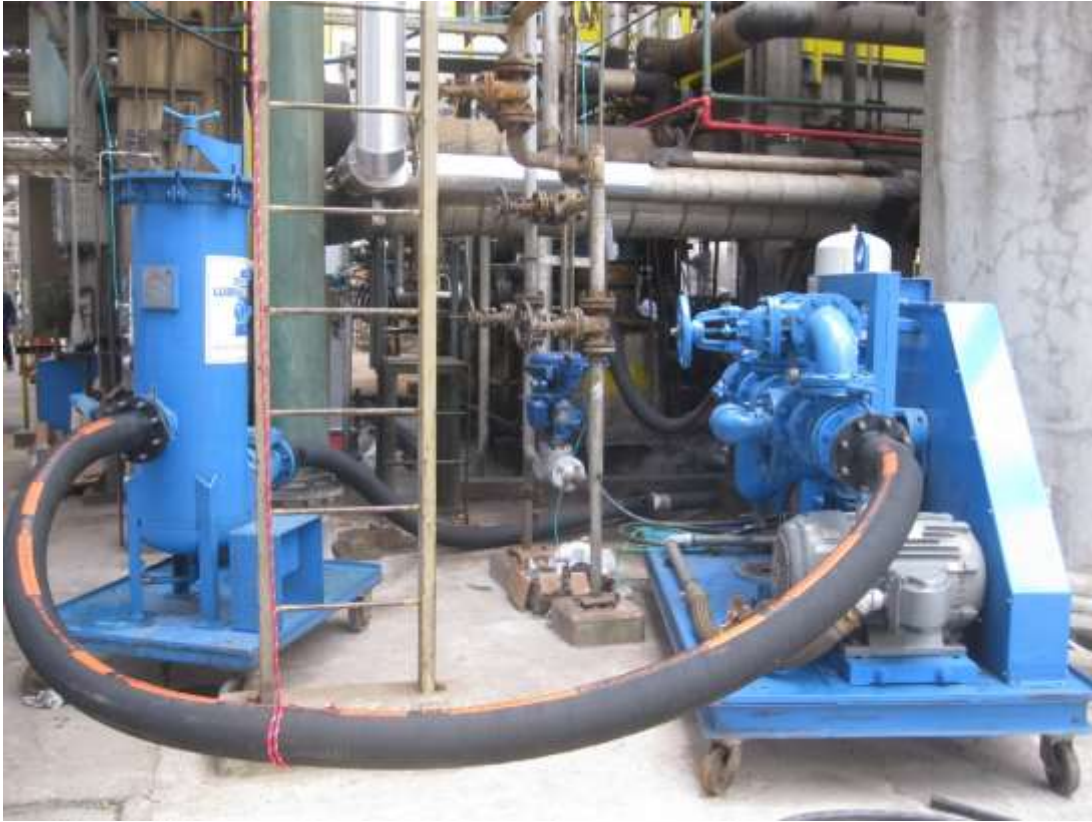
Flushing skid with positive displacement pump at 500 GPM flow and filter housing with four 34" filter elements.
